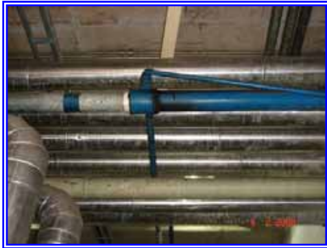
Main Air Supply
