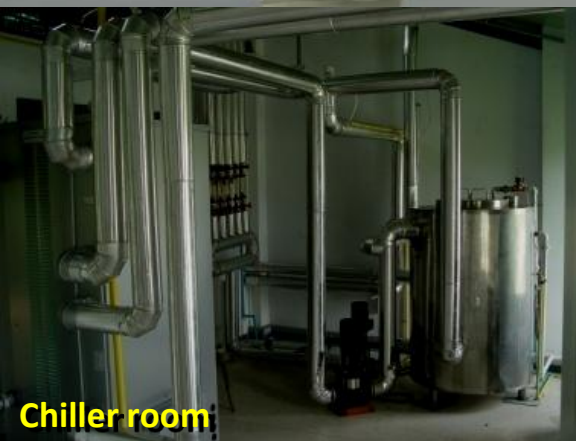
Testing Building with Solar Cooling System
