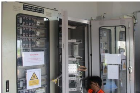
Generator Control Panel
