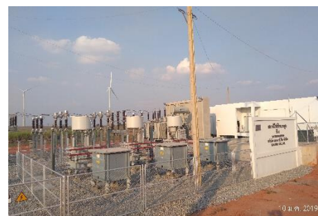
SUB STATION 115KV
